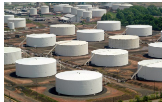
Petroleum Product Tank Farm
